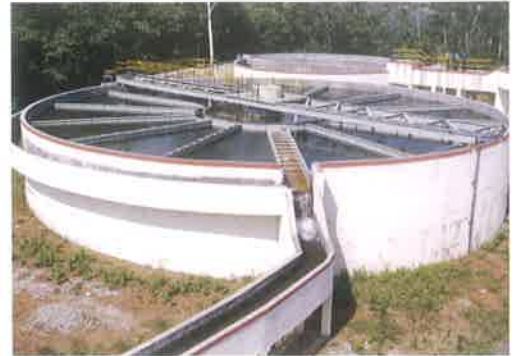
40 MLD WTP, Curti-Ponda , PWD, Goa
