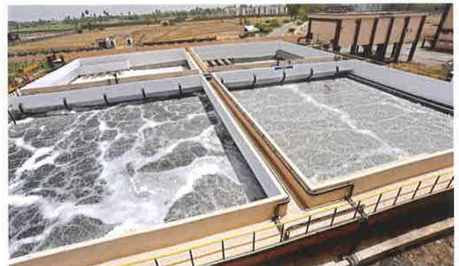
MBBR Unit at 84 MLD STP, Variav for Surat Municipal Corporation
