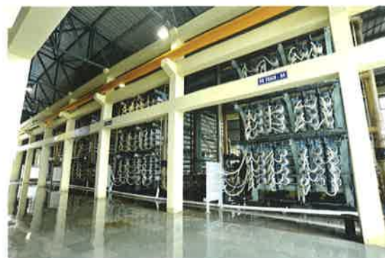
Reverse Osmosis System
