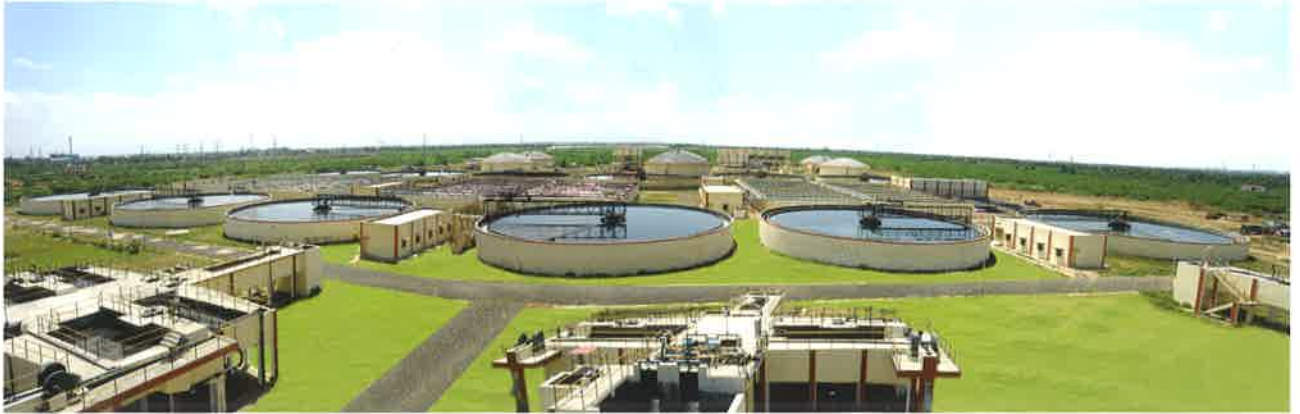
180 MLD STP, Pirana, Municipal Corporation, Ahmedabad India's First Largest STP with Diffused Aeration and PLC -SCADA System
