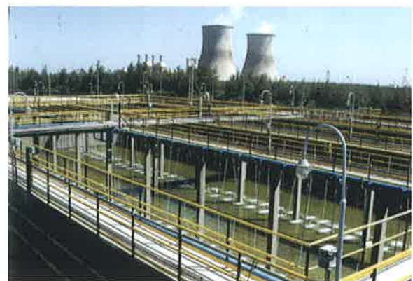
Diffused Aeration based Effluent Treatment Plant including Tertiary Treatment for reuse of waste water for Reliance, Hazira
