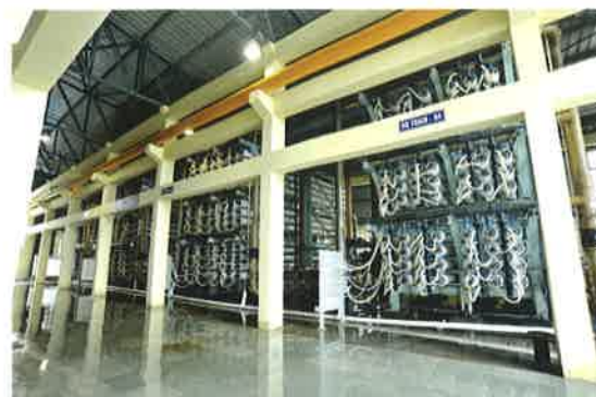
Reverse Osmosis System
