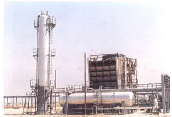
Effluent Treatment Plant for IFFCO-Aonla
