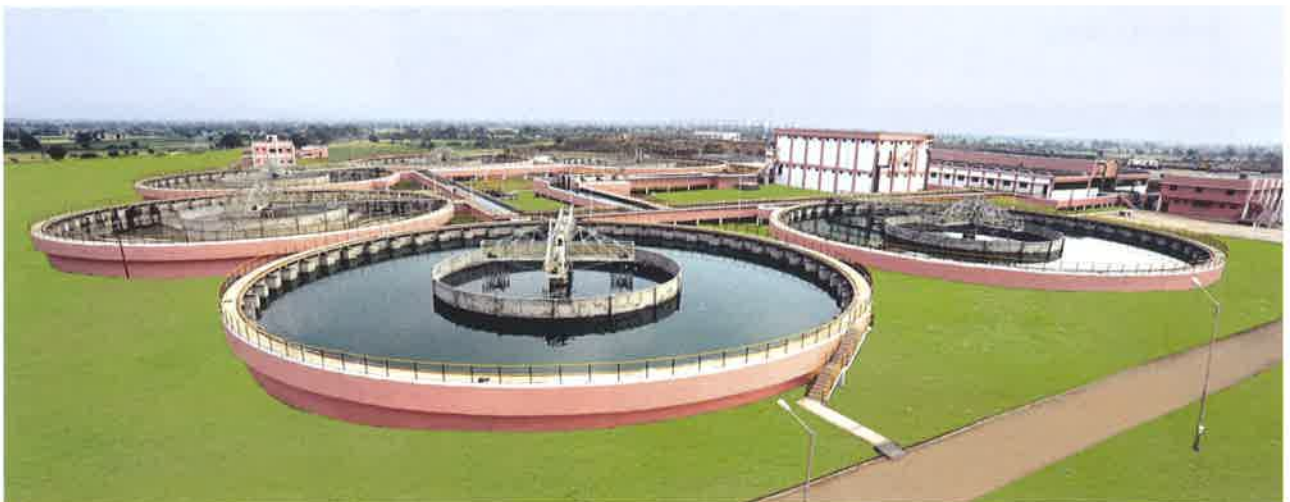
363 MLD, WTP at Baklai for Indore Municipal Corporation
