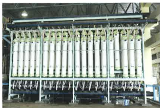
Ultra Filtration System
