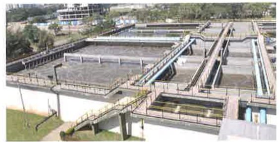
SBR Unit at 40 MLD STP at Kharadi, Pune
